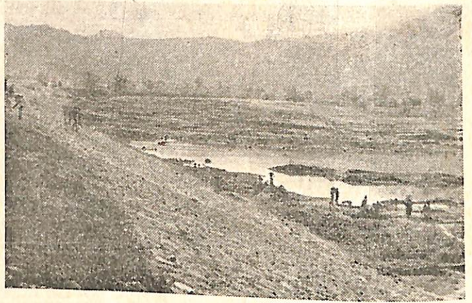
Construction of earth dam of Dumerjore M. I. P. of Nawapara Subdivision.
