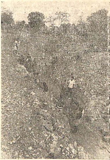
Construction of earth dam of Armela M. I. P. in Nawapara Subdivision
