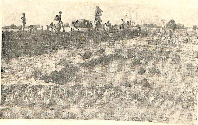
Construction of earth embankment of Budhikomna M. I. P. in Nawapara Subdivision.
